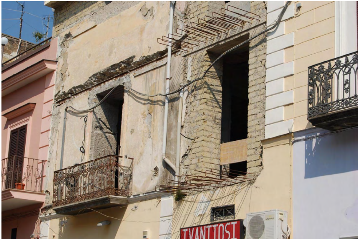
Fig. 2: Sarno (SA), inner-city. Still today it's ordinary to substitute "traditional" building components with incompatible materials and features.
