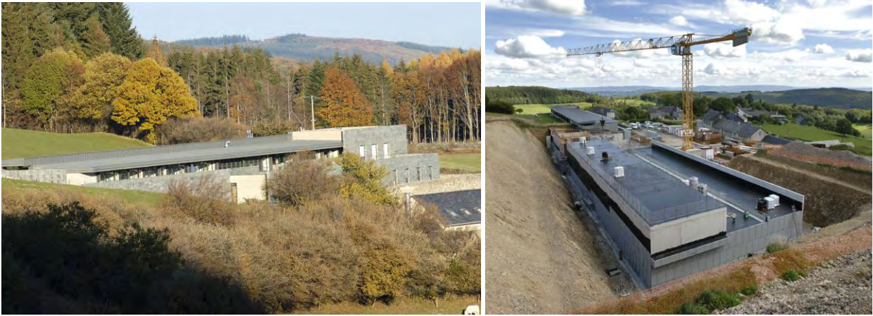
Fig. 4: The Centre archéologique européen , with the construction site of its extension devoted to the central store of archaeological finds from Burgundy (architect: Pierre-Louis Faloci ; Antoine Maillier ©Bibracte)
