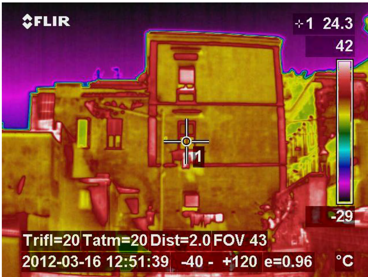
Fig. 9: Sarno (SA), sample block, inner southern front. The thermography IRT proves the masonry stratigraphy.
