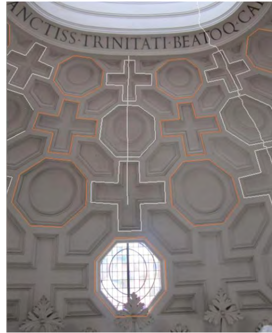
Fig. 8 Photo which show the octagonal and cross coffers and overlay of photogrammetric survey
